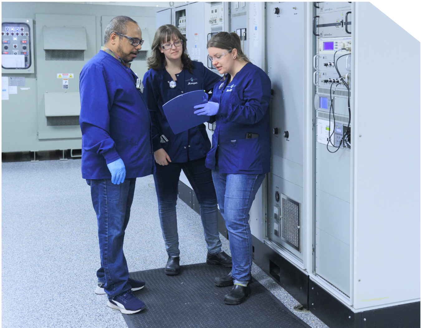
Figure 6 – Fedoruk Centre Technologists at the cyclotron power system.
